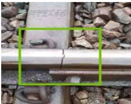
Fig 1: Railway Track Crack
